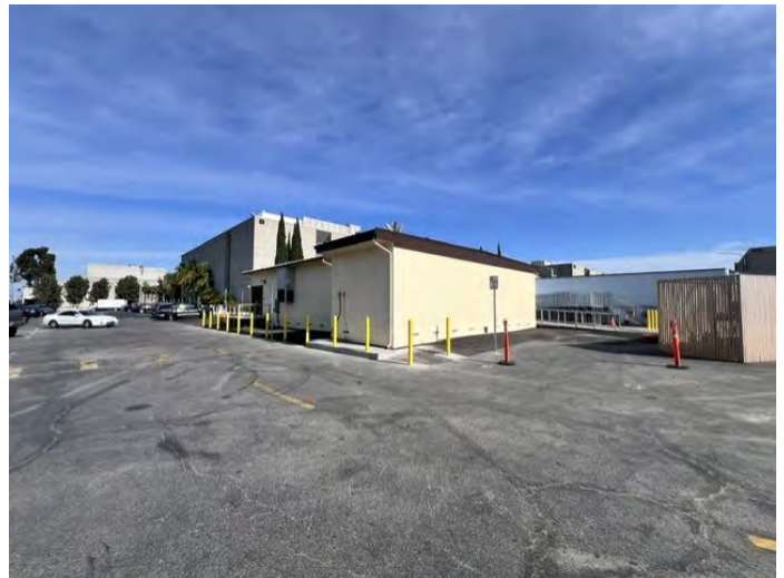
Swing Space—Hotel, Restaurant, and Culinary Arts: Kitchen, and Restroom and Dining Room—Modular Construction Activities
