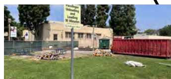
Wilshire Chiller Plant Relocation [Construction]
