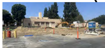
Wilshire Chiller Plant Relocation [Construction]
