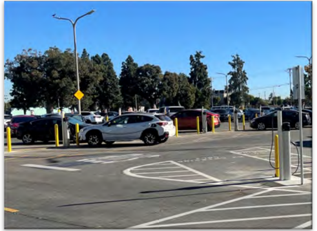
Electrical Vehicles (EV) SCE Charging Stations — Completed Stations
