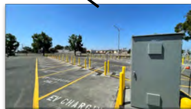
Electrical Vehicles (EV) SCE Charging Stations-Lot 4 [Close-Out]
