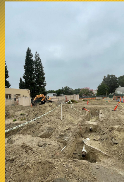
Unforeseen Telecom Duct Bank
