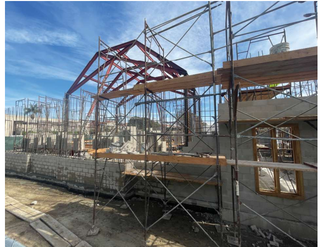
New Performing Arts Complex Concrete Masonry Unit Installation and Scaffolding at West Building Recital Hall
