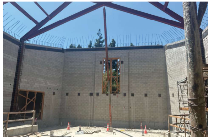
New Performing Arts Complex Steel Structure and CMU Walls in West Building Recital Hall
