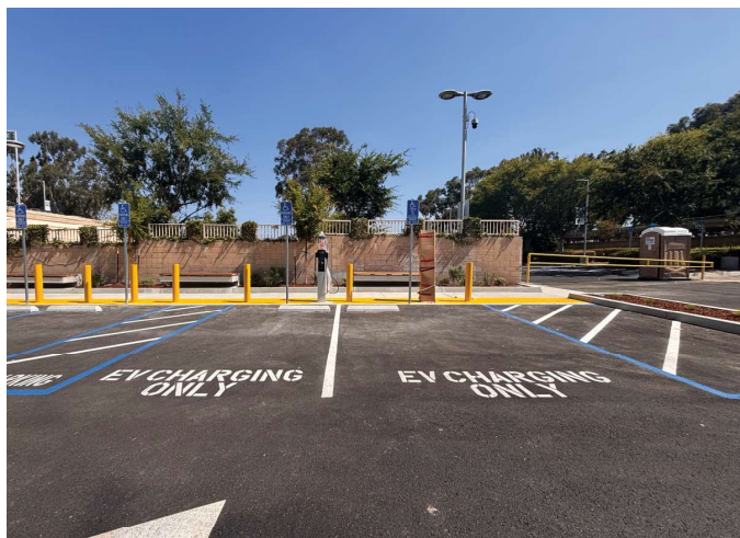
Restore East Parking Lot Installed Electrical Vehicle Charging Stations
