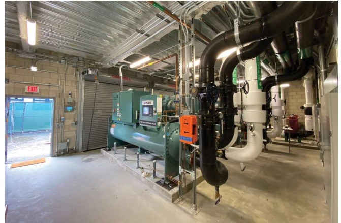
Wilshire Chiller Plant Relocation Completed Site
